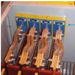
Bus bar transits for transformer room.
