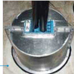
Transits for submarine cable in foundation.
