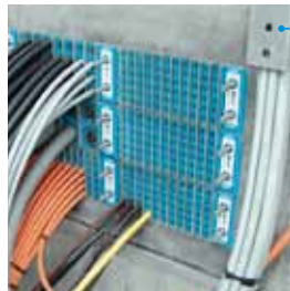
Transits for substations.
