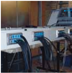
Transits for potential equalization, and standard system for control cabinets in the nacelle.
