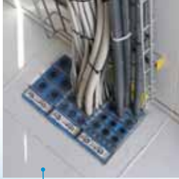
Transits between fire zones in offshore substations.
