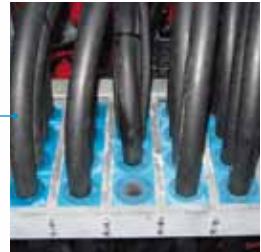
Retention systems below nacelle and in tower.
