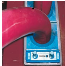
Roxtec S frame with power cables for generator sets.
